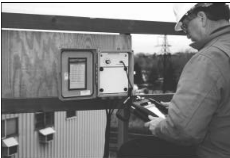
Figures 10 - Accessing data from switch box.
