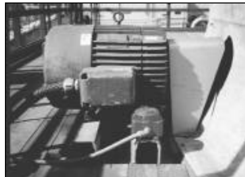
Figure 3 - Cooling tower motor.
