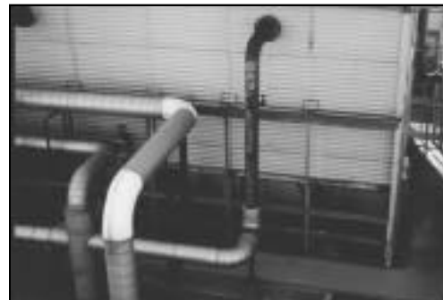
Figure 4 - Cooling tower pool (located under the tower structure).
