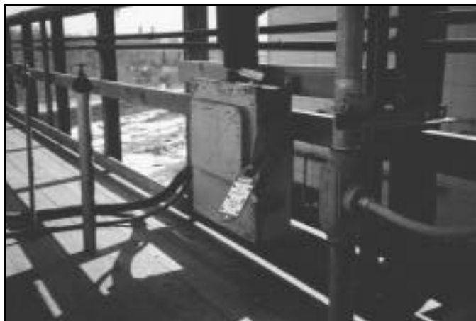
Figure 6 - Lock-out of cooling tower fan during accelerometer placement.
