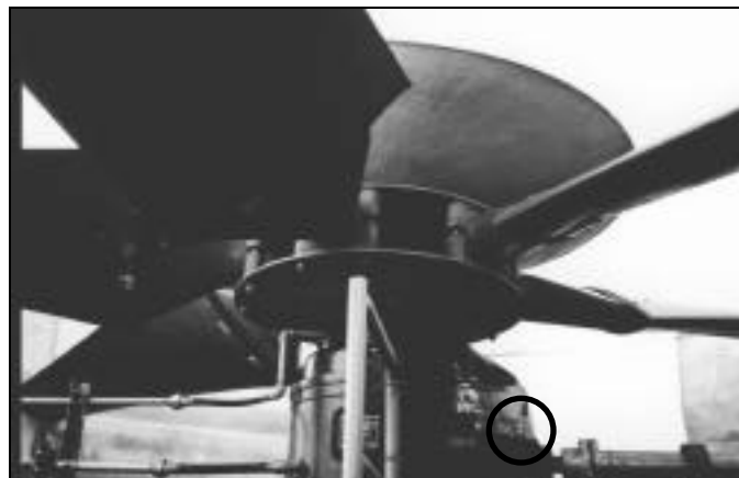
Figures 8, 9 - Permanently mounted accelerometers.
