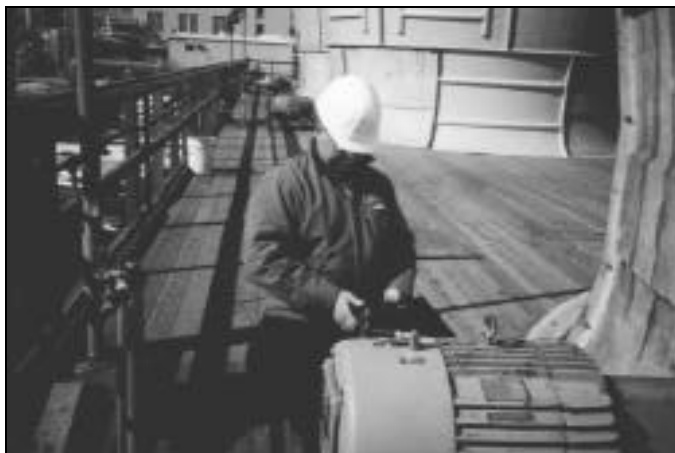
Figure 5 - Portable collection of vibration data from cooling tower motor.
